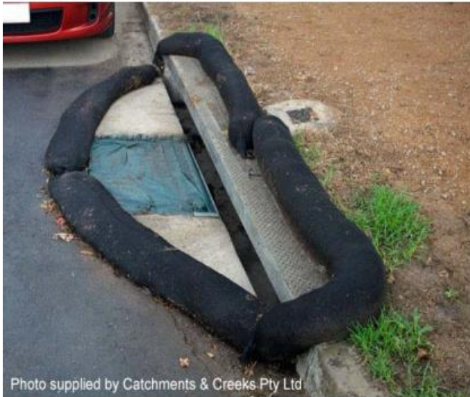
Figure 9: Use of filter socks to form a sediment trap at sag inlet
