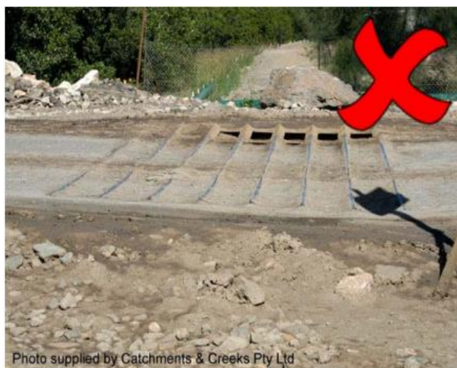
Figure 2: Lack of maintenance resulting in heavy sedimentation
